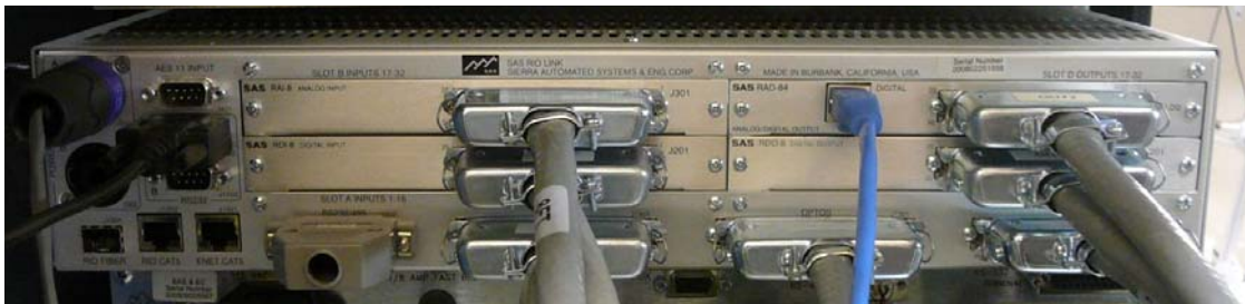
RIO DSP ENGINE With RJ32 Cabling to Punch Blocks (Typical)
